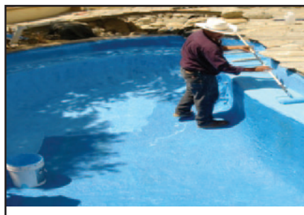
2ND COAT OF "THE BLUE STUFF" BROADCAST 16-20 SILICA SAND WHILE STILL WET
